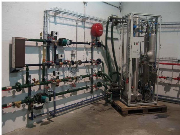
Figure 4: Test stand for the absorption chiller at Pink (Source: Pink)
