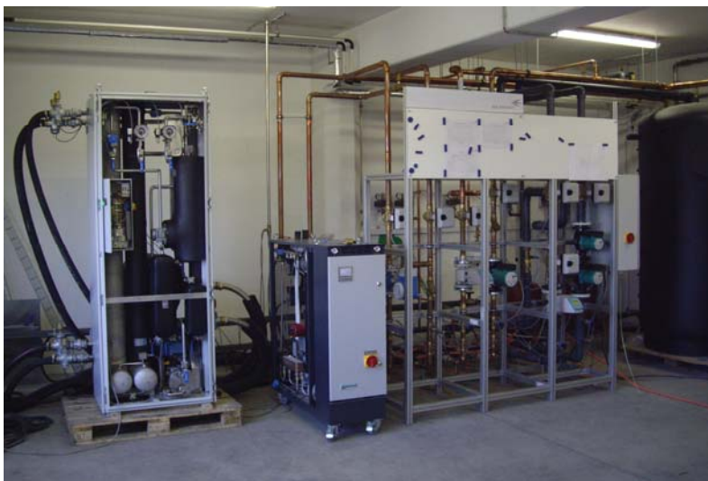
Figure 3: Test Stand at SolarNext with the absorption chiller (Source: SolarNext)
