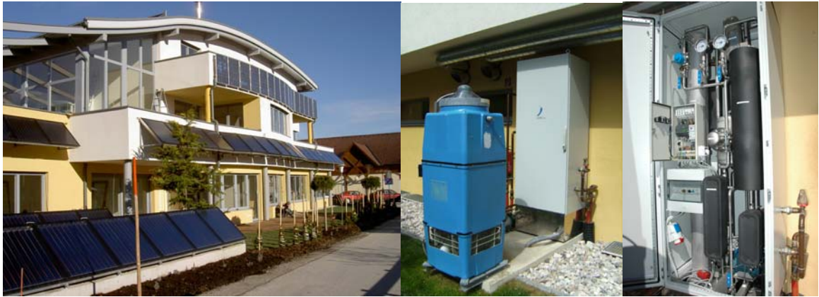
Fig. 6. Flat plate collectors on the facade and the ground as well as absorption chiller chillii ® PSC10 at the training center and office building of the company BachlerAustria (sources: SolarNext).
