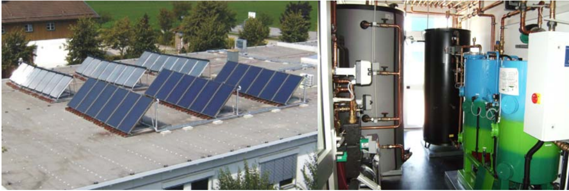
Figure 5: Flat plate and vacuum tube collectors on the roof of the SolarNext provide the chillii® solar cooling and heating system, the heart of the system is an EAW Wegracal SE15 (sources: SolarNext)
