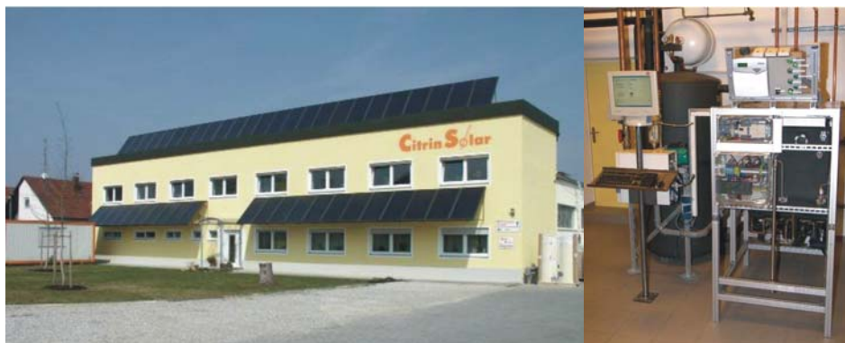
Figure 1: Solar air-conditioning system of CitrinSolar with flat plate collectors on the façade and on the flat roof as well as the chillii ® STC6 adsorption chiller (sources: CitrinSolar)
