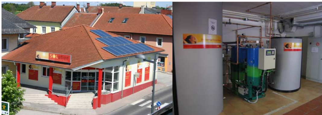
Figure 6: Flat plate collectors on the roof and EAW Wegracal SE 15 absorption chiller in the technical room of Sol-ution in Sattledt, Austria (source Sol-ution, EAW)
